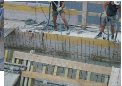
Compacting concrete in a building, using electric internal vibrators from the NCZ series
